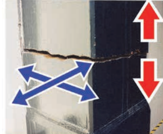
柱の破断 (1985 Kobe Earthquake) Sudden fracture of many steel columns
